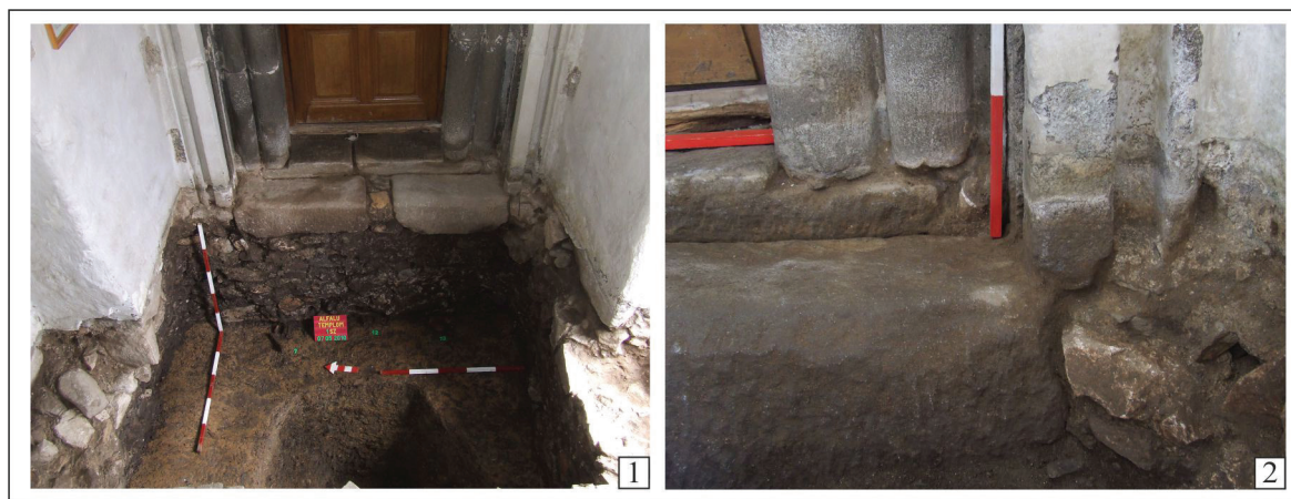
Fig. 4. 1. Joseni. Final ground of S1; 2. Detail with the placement of the frame on the threshold and the tower foundation.
